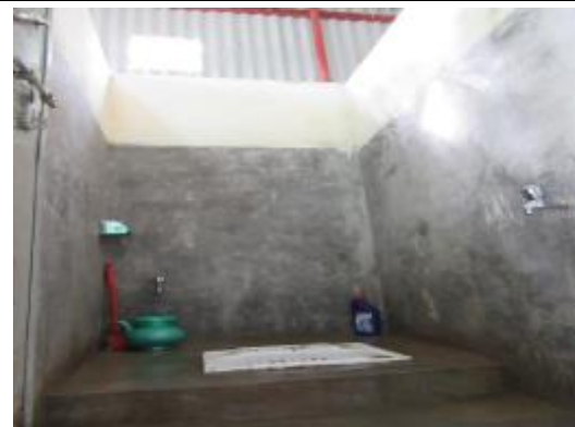
NDE Employees' Labor Shed Sanitary Conditions
