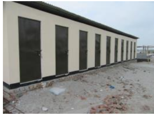
Toilet Facilities of Subcontractor Labors Sheds of NDE
