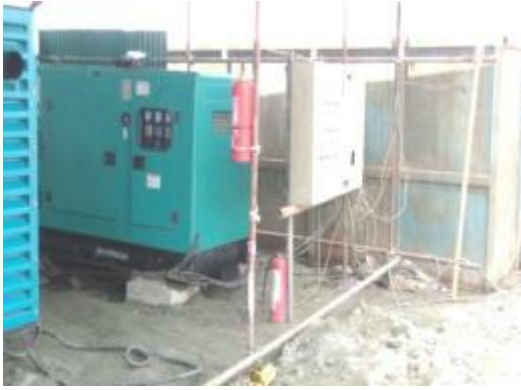
Fire Extinguisher in Project Site
