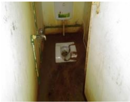
Irregular Cleaning In NEPC Subcontractor Labors' Sheds
