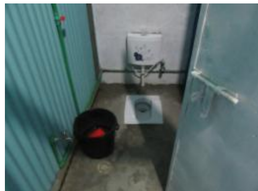
Toilet facility (NEPC)
